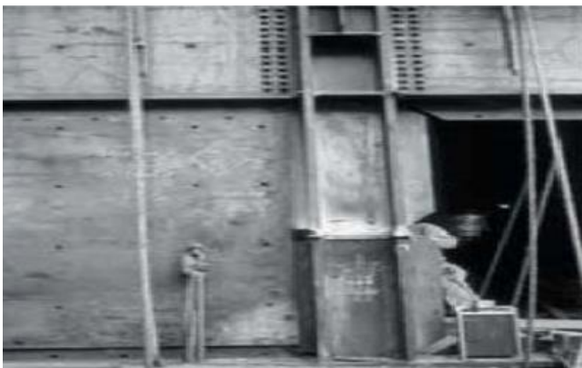
Fig 2. An example of a steel shear wall worked in a hotel in Dallas, Texas.
